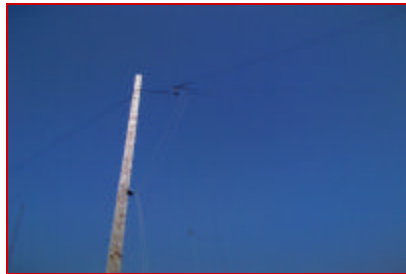
ISSUE #2 - A new element being hoisted into place to be connected to terminator and feed lines.
