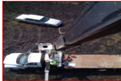
Shot taken from the crane basket by Jason Cooper inspecting the work.
